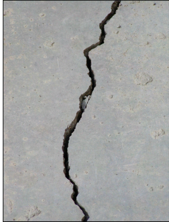
Fig. 4 Close-up View of Example Floor Slab Crack
