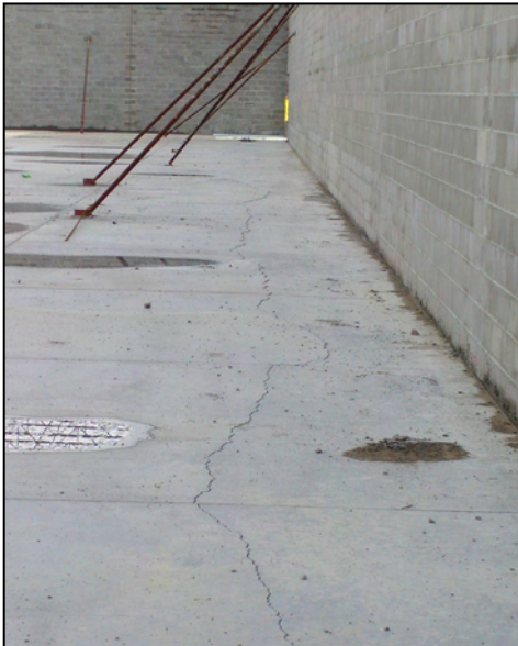
Fig. 3 Example Floor Slab Crack Adjacent to South Wall
