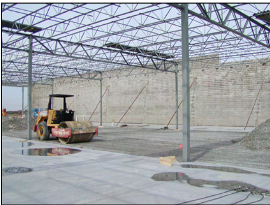
Fig. 7 View from Inside Target Store
