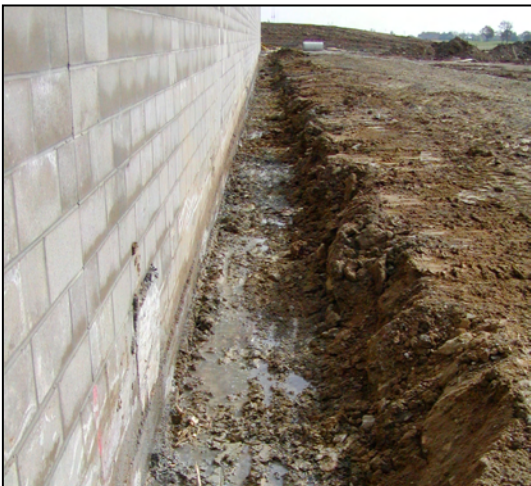
Fig. 8 As-Built Spread Footing Shown Nearly Flush with Exterior Wall
